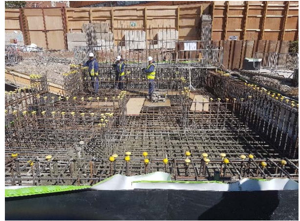
Concrete being poured to the main tower containing the central stair and lifts
